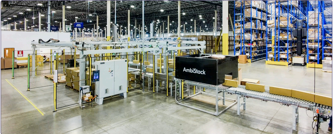
*AmbiStack dual system configuration installed at customer facility
